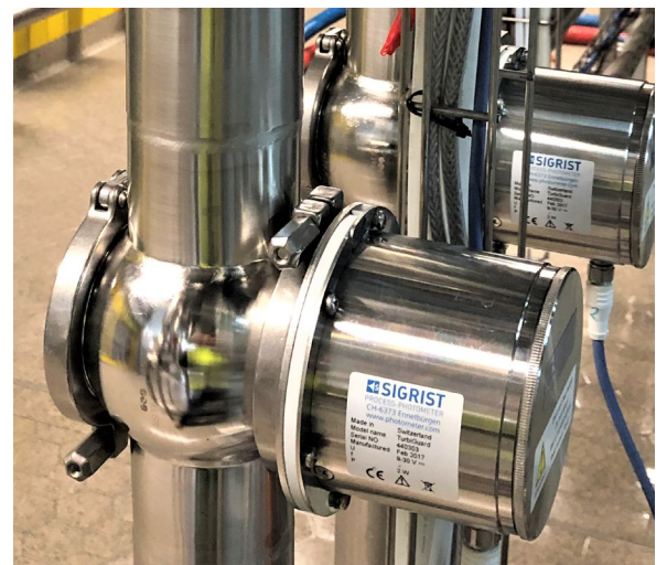
Figure 2: Transfer pipes with TurbiGuards installed inline
