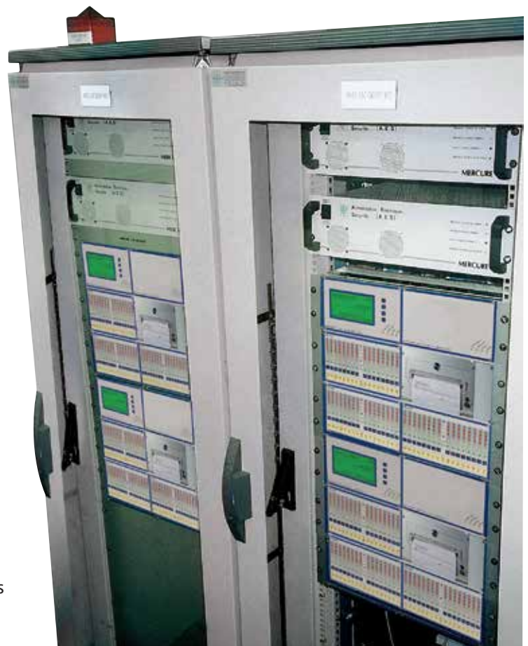
Example of installation with 256 detectors
