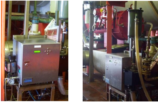
Picture 4: OilGuard installation on an oil platform
